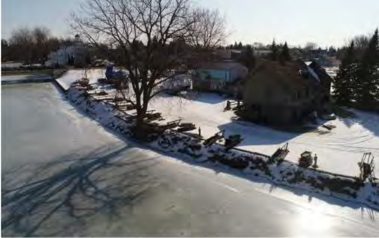
PHOTO 3: FISHING PIER, PROMENADE AND PICNIC AREAS The drone's camera faced south-east for this photograph. Four-hundred and twelve feet of steel sea wall will support the creation of a concrete promenade and shore fishing pier. LED bollard-style lighting along the promenade will be consistent with the landscaped, minimizing light pollution, and supporting longer use of the picnic areas around the park's UD pathways. (2/2020)
